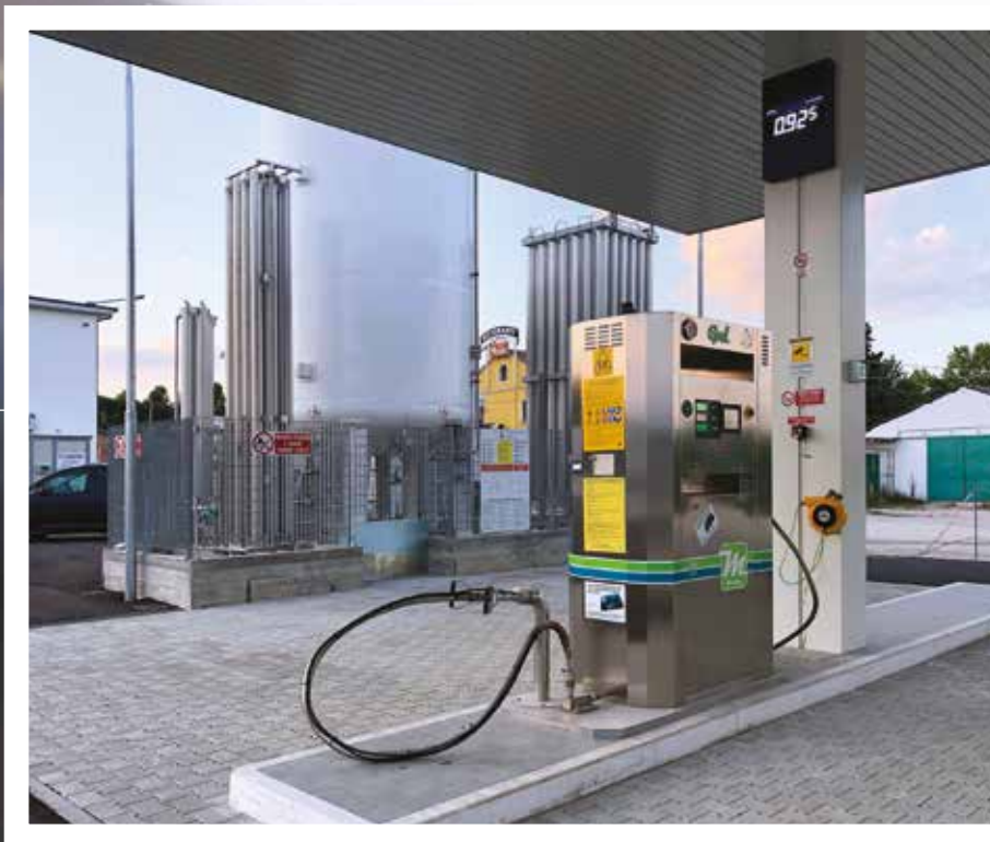
Q8 plant built by Ham Italia in Roseto degli Abruzzi (TE).
